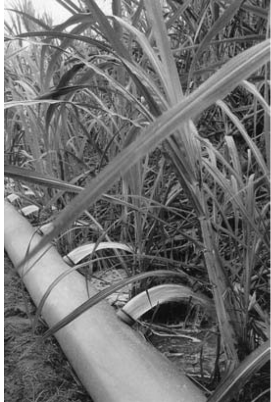
Fig. 5.9 Typical fluming system in Queensland, Australia. Source: C. E. Bartlett Pty Ltd, Australia.
